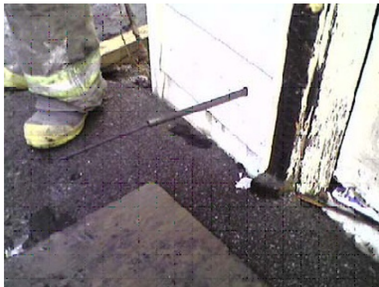
Photo from Hillcrest Fire
