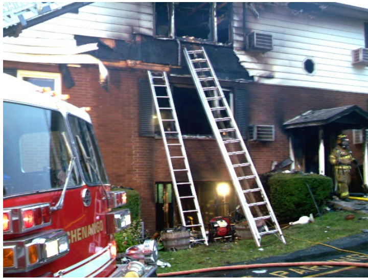
Fire Damage on Side A of the apartment building.
